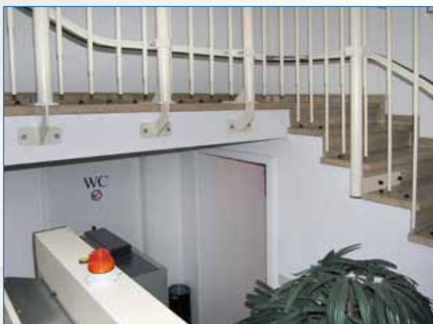
Guide rails fixed with a combination of posts fixed to the flank of the stairs, and struts in front of the risers
