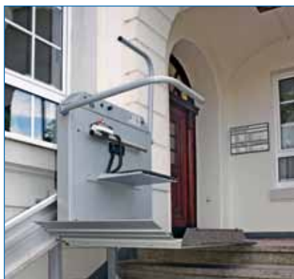
HIRO 350 at the upper landing, ready for access
